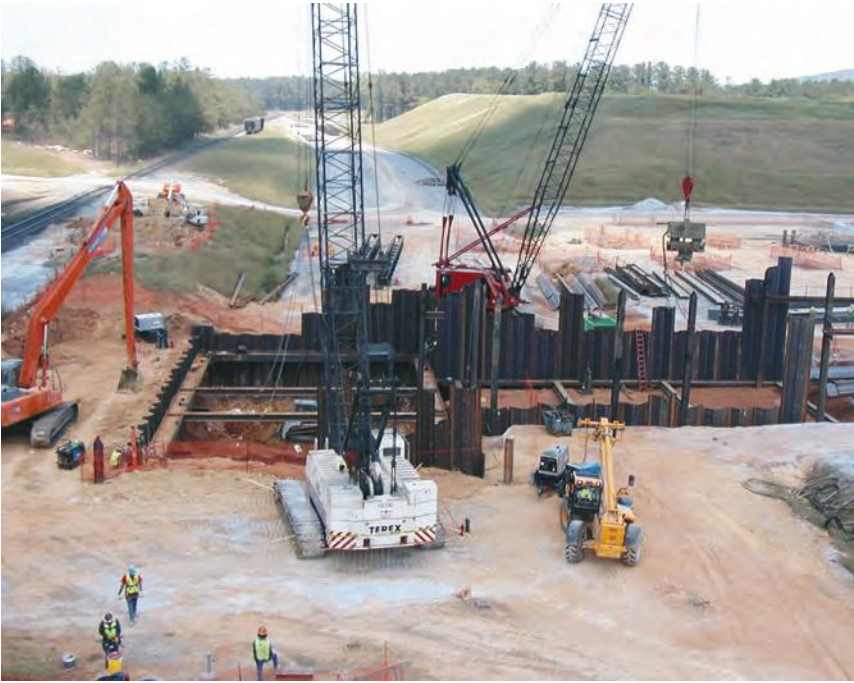
Sheet piles and interior bracing for rail unloading (left) and conveyor tunnel (right).
