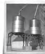
OVERHEAD WEIGH HOPPERS
