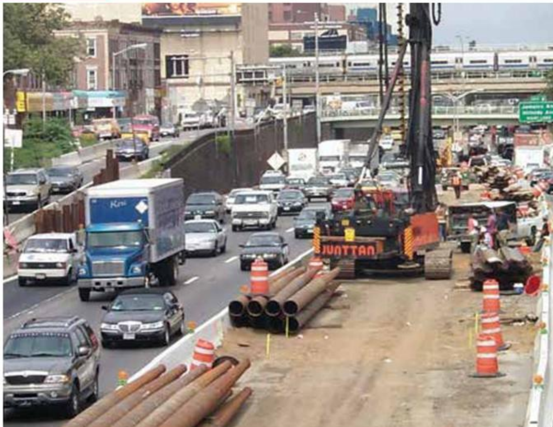
TAPTUBE PILES in use for the JFK Light Rail project being installed at NYC Van Wyck Expressway
