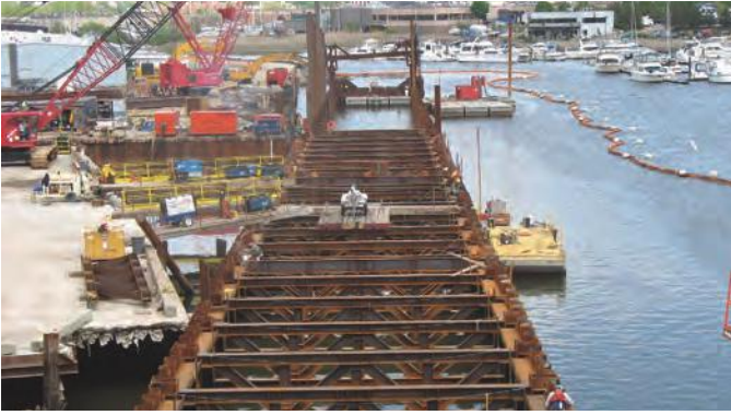
Dura-Bond supplied the fabrication provided the seal welding on sheet and king piles for Mystic River project.
