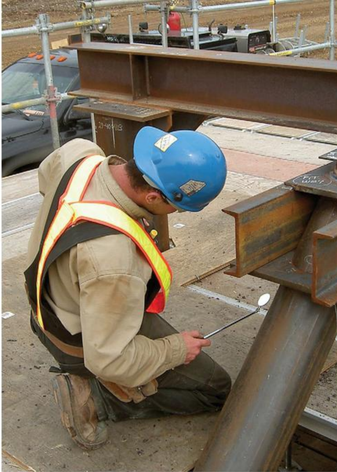
TFL offers on-demand, mobile welding services, including pile splicing and pile capping
